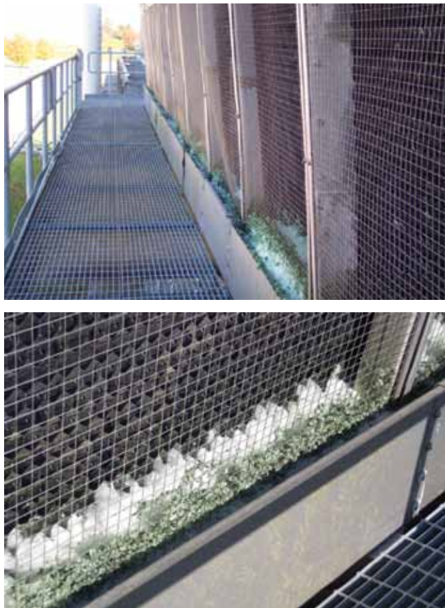
Figure 4: Foamy sump at Field Study #1
